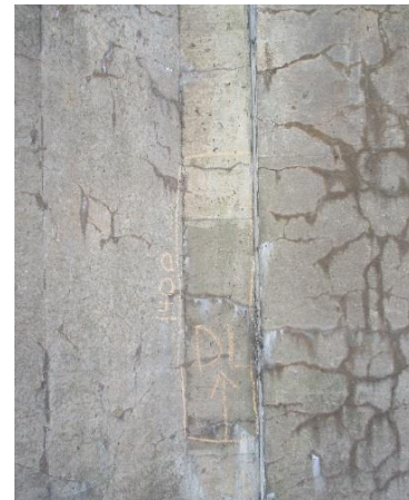
Figure 6: Delamination on south abutment.
