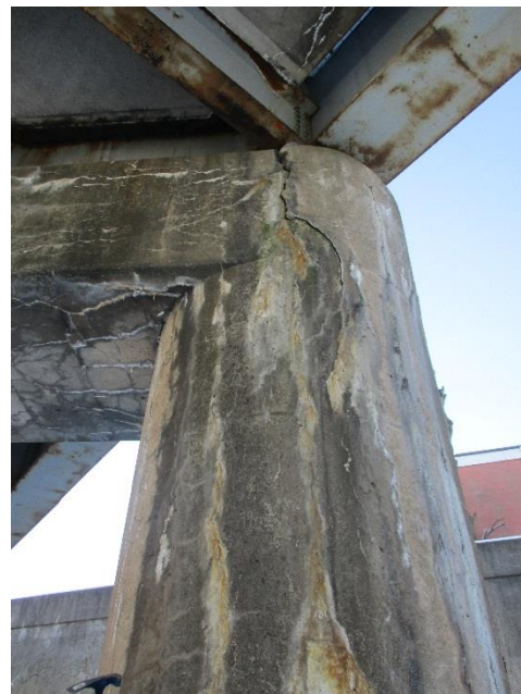
Figure 8 - Cracking on the northwest pier.
