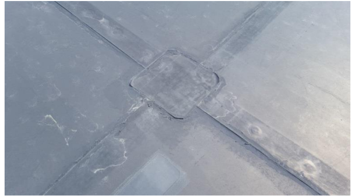
Photo B.38 – Original cover at seam intersection.
