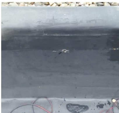
Photo B.41 – Exposed flashing screw holes in EPDM.
