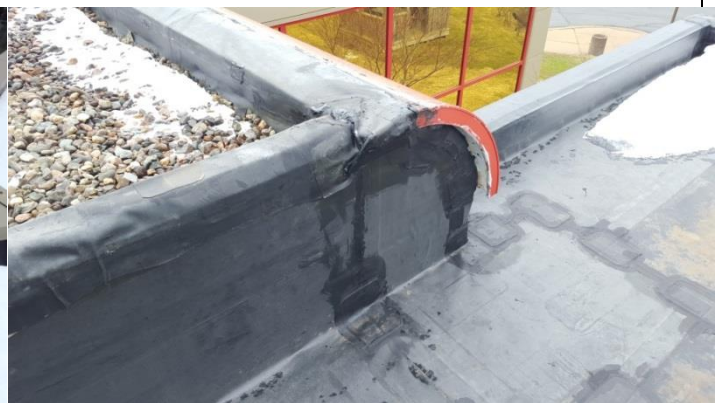
Photo B.36 – Cap flashing removed at entrance.
