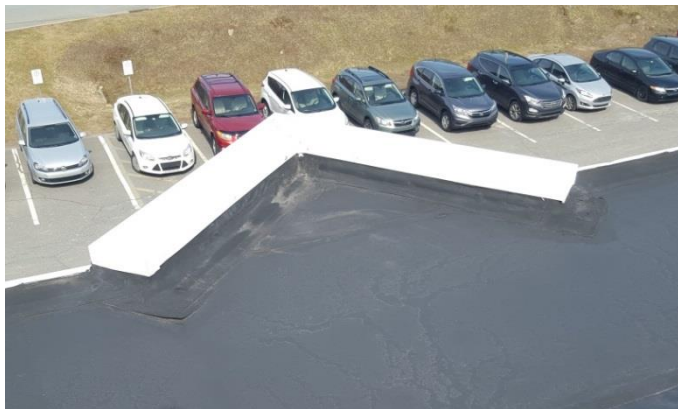
Photo B.5 – West facing parapet with lifting flashing.
