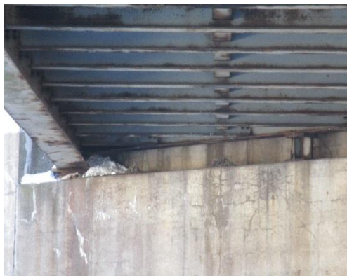
Figure 10: Snow collecting on south beam seat.
