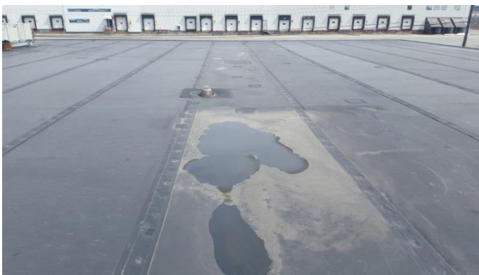
Photo B.65 – Standing water, northeast corner.
