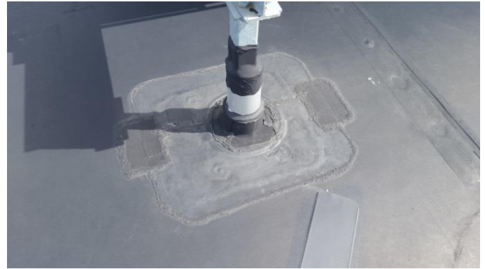
Photo B.50 – Typical boot at AHU support.
