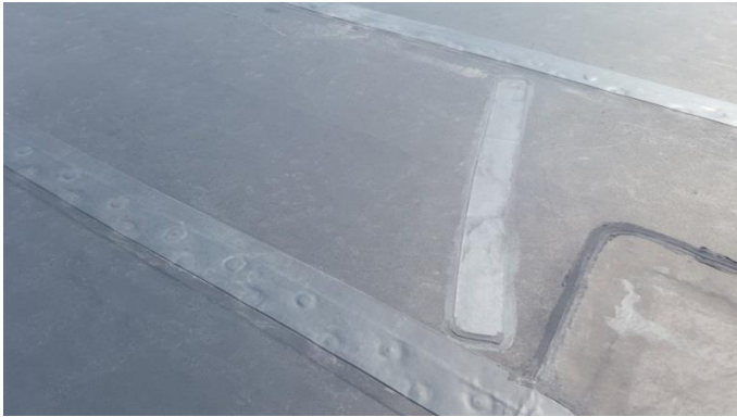
Photo B.7 – Typical seam-damage patches, west.
