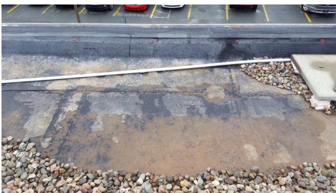
Photo B.11 – EPDM membrane tenting edge.
