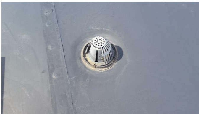
Photo B.33 – Broken aluminum strainer dome.
