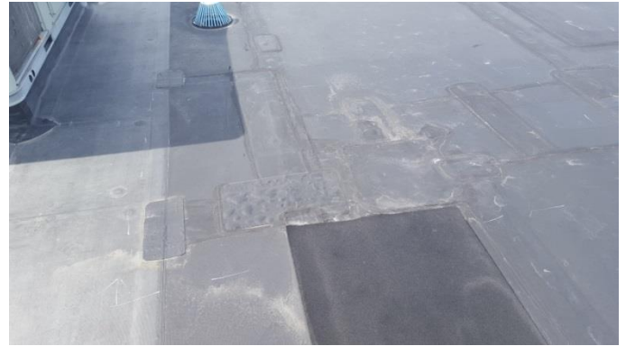
Photo B.26 – Wear mat and adjacent patching.
