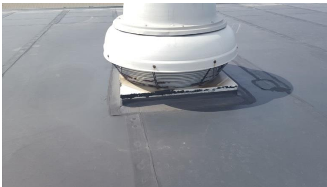
Photo B.45 – Low curb at fan penetration.
