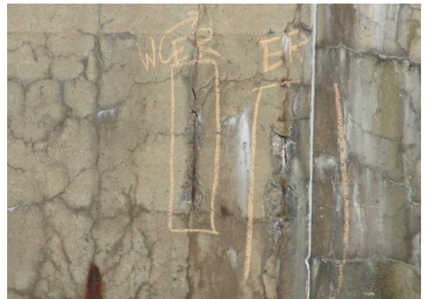
Figure 4: Close up of exposed rebar.
