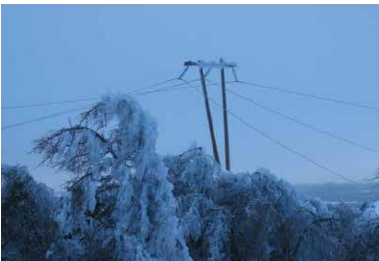
Storm related damage caused by freezing rain in Newfoundland. Photo courtesy of Newfoundland Power Inc.
