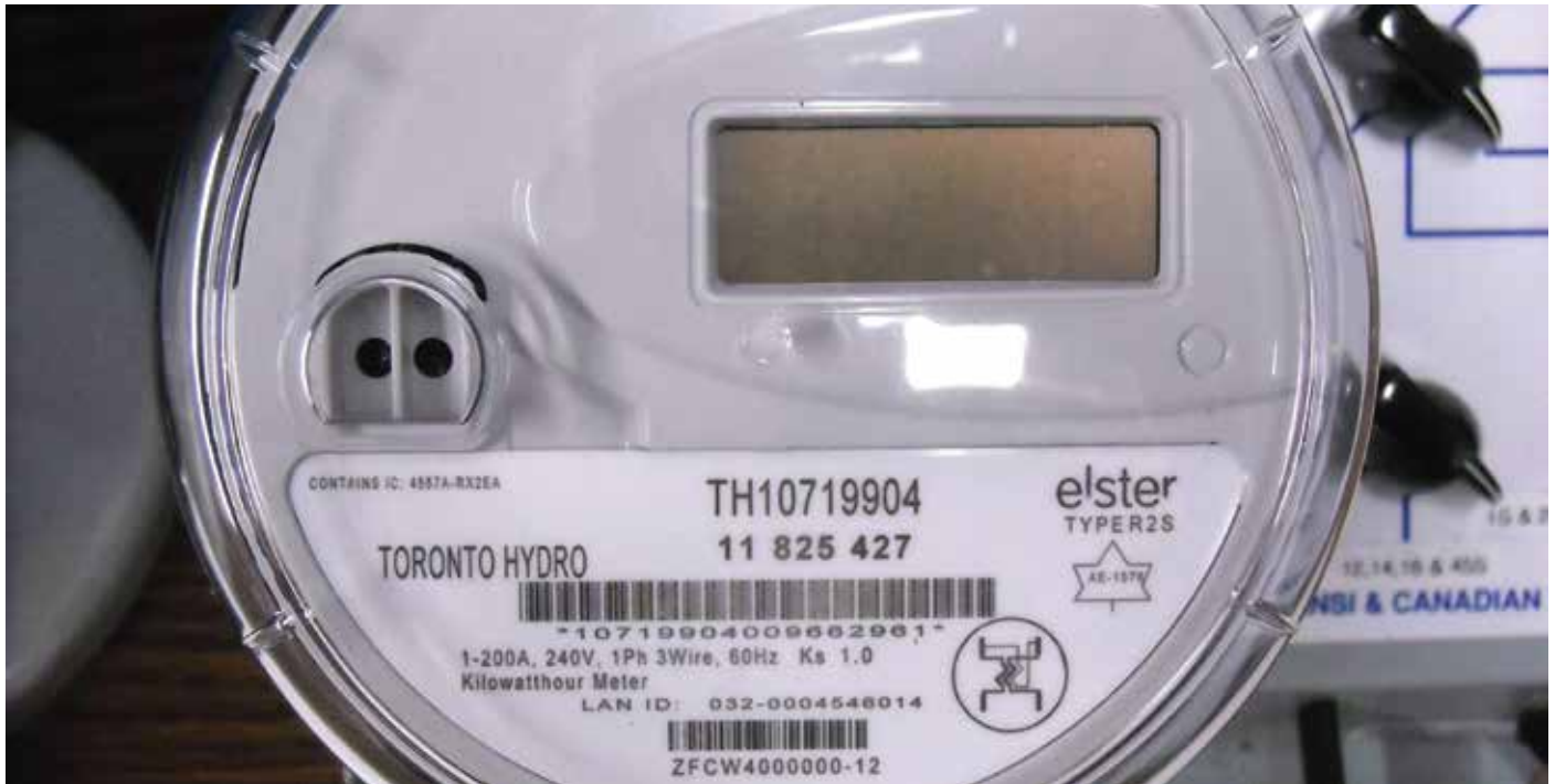
Toronto Hydro Corporation has converted 99.7 per cent of its meter population to Smart or Interval Meters. Photo courtesy of Toronto Hydro Corporation.
