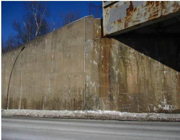
Figure 3: North abutment delamination and exposed rebar.
