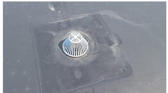
Photo B.64 – Roof drain with broken plastic strainer.
