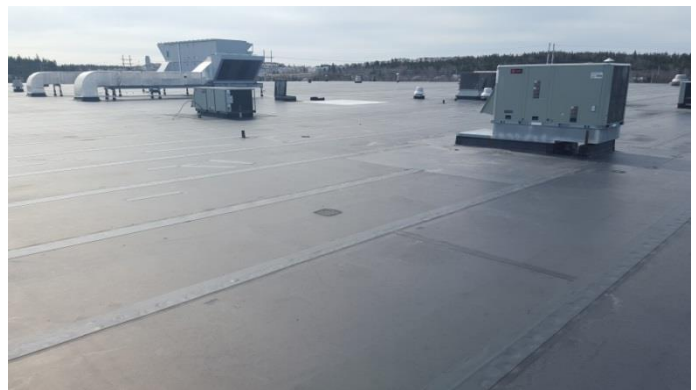
Photo B.18 – View of mechanical, looking southeast.
