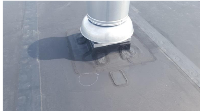
Photo B.8 – Vent penetration with patching/repairs.
