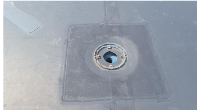
Photo B.62 – Roof drain with missing strainer dome.
