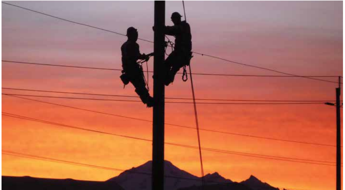
BC Hydro power line technicians work to ensure power. Photo courtesy of BC Hydro and Power Authority.
