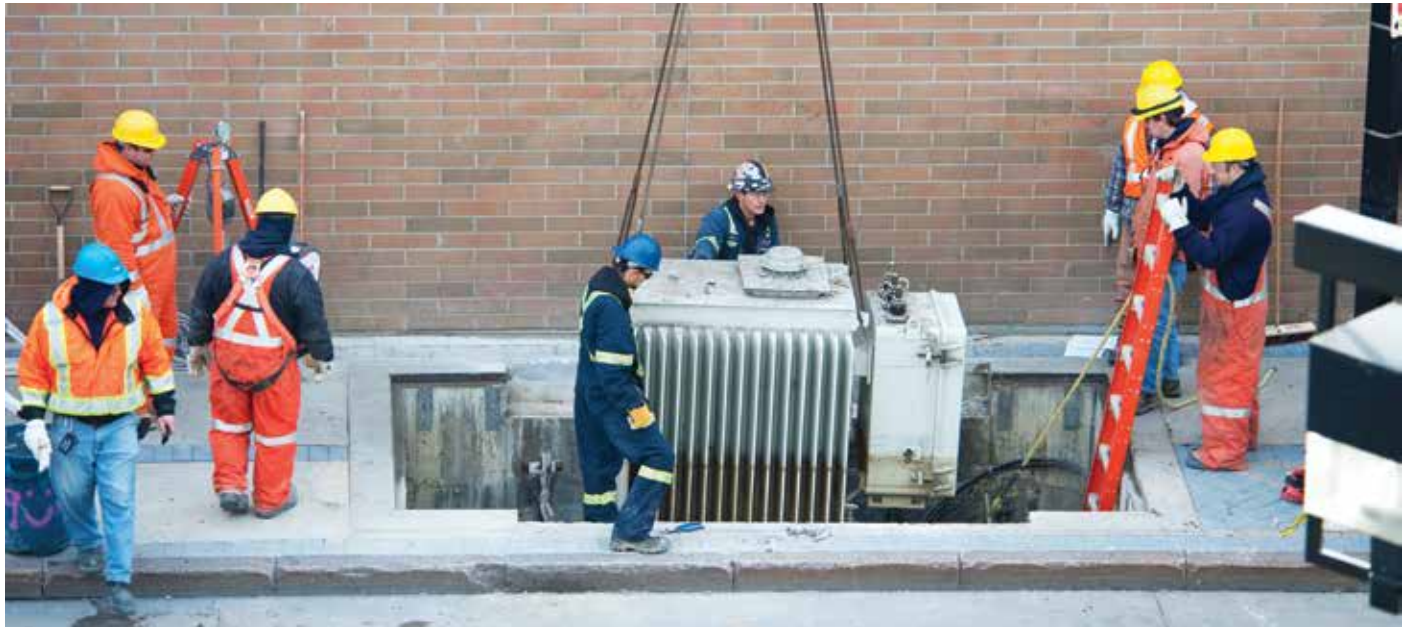
Manitoba Hydro crews install new equipment in a vault beneath Graham Avenue in downtown Winnipeg as part of the utility's infrastructure renewal efforts. Photo courtesy of Manitoba Hydro.
