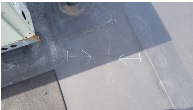
Photo B.41 – Noted failures from previous
