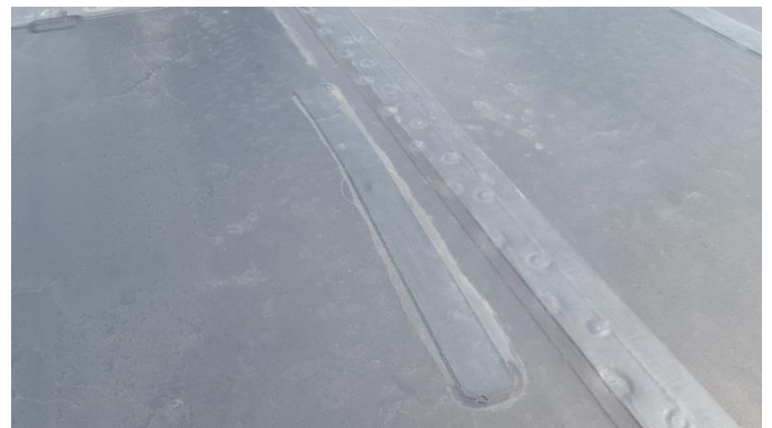
Photo B.10 – Patching at seam and damage.
