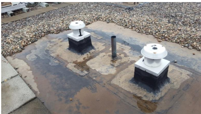
Photo B.29 – Exposed membrane at penetrations.
