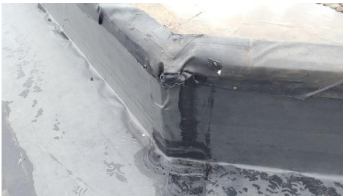
Photo B.39 – Exposed membrane joint.
