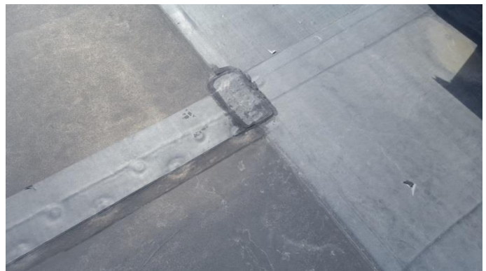
Photo B.12 – Patch with joint cover strip.
