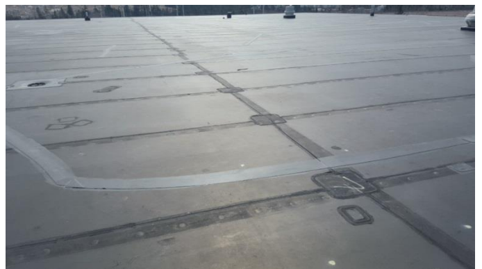
Photo B.48 – Patch lifting, drain strainer missing.
