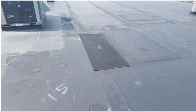
Photo B.25 – Patches at seams and in roof field.
