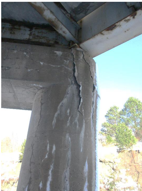
Figure 7: Cracking, delamination, and spalling of concrete on southeast pier.
