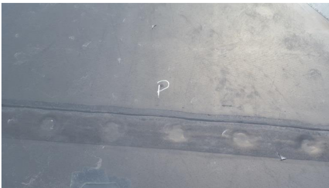
Photo B.63 – Unpatched perforation at fastener.
