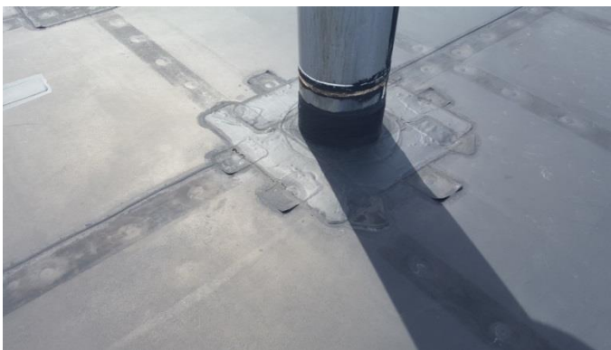
Photo B.59 – Adhesive failure at penetration flashing.
