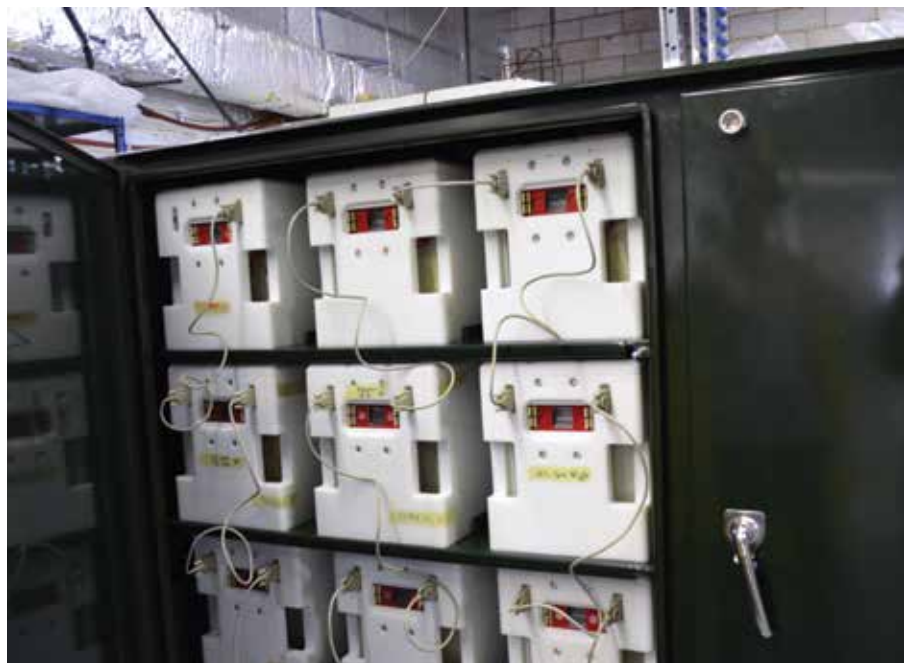
Toronto Hydro's community energy storage system was developed with a lithium-ion battery solution used for distribution grid applications. It consists of batteries, controls, and communication systems that interface with the grid and was made possible through funding in innovation. Photo courtesy of Toronto Hydro Corporation.
