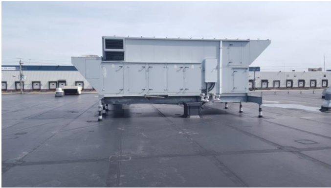
Photo B.49 – Air Handler, close to north roof edge.
