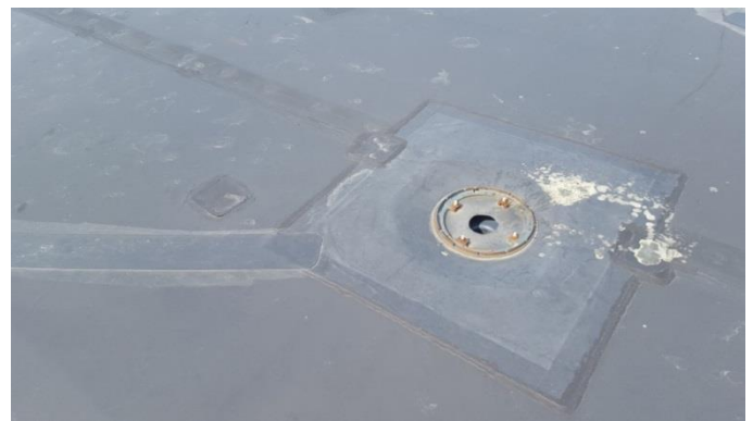
Photo B.54 – Roof drain with missing strainer dome.
