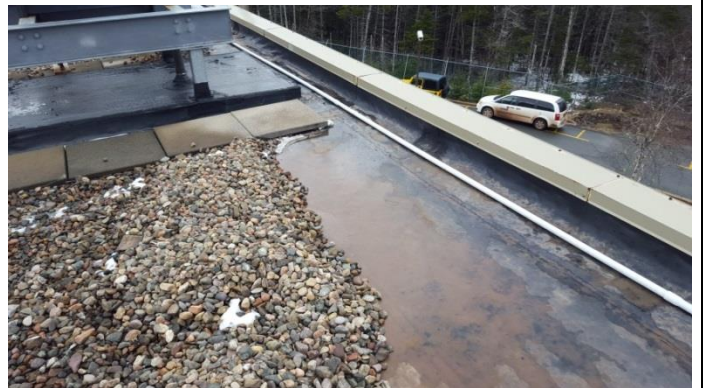
Photo B.28 – Ballast and water buildup at new unit.
