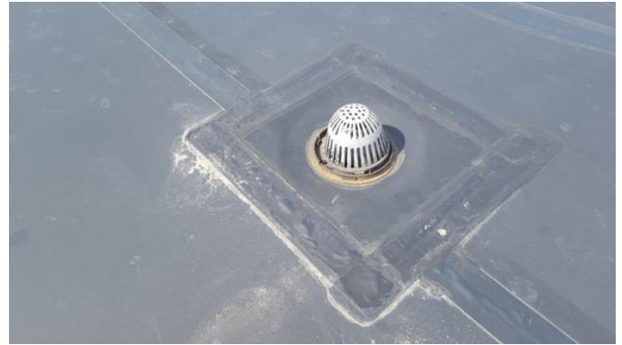
Photo B.56 – Damaged aluminum strainer dome.
