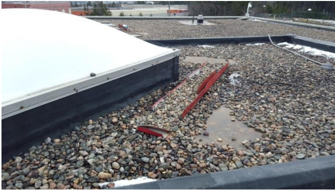
Photo B.37 – Flashing stored on roof using ballast.
