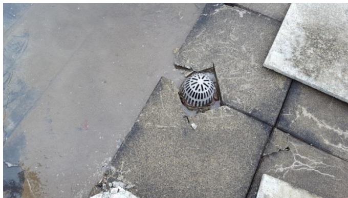
Photo B.23 – Broken pavers on membrane.
