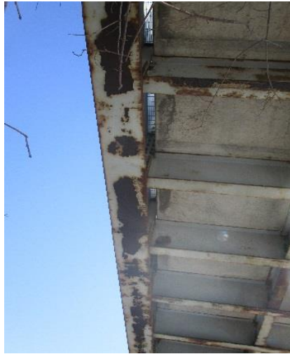
Figure 12: Peeling of paint on south girder.
