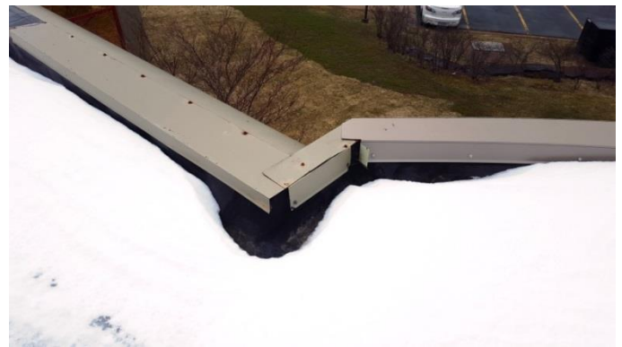
Photo B.34 - Note flashing condition (poor jointing).
