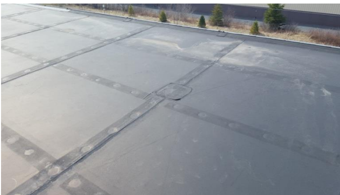
Photo B.35 – Failing EPDM patch and seams.
