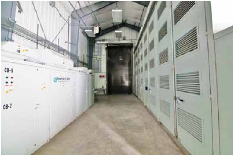
A view of the interior of BC Hydro and Power Authority’s Field energy storage facility. Photo courtesy of BC Hydro and Power Authority.
