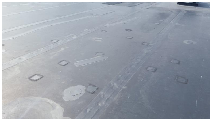
Photo B.24 – Patches and standing water stains.
