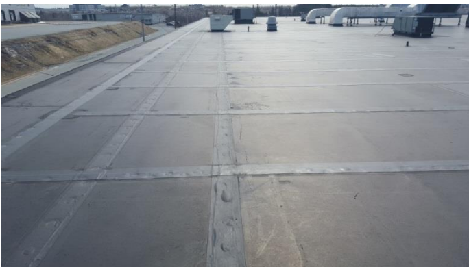
Photo B.17 – Note blistering in seam cover strip.
