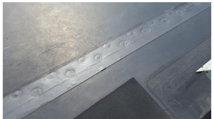
Photo B.42 – Seal failing on edges of seam cover.
