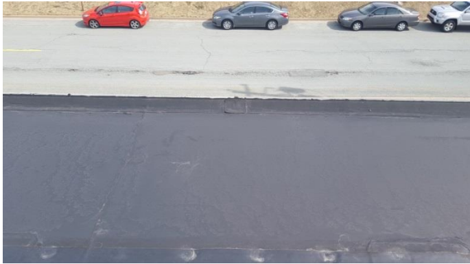
Photo B.19 – Edge flashing patch failure.
