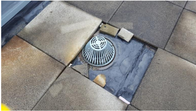
Photo B.19 – Pavers broken and resting on EPDM.
