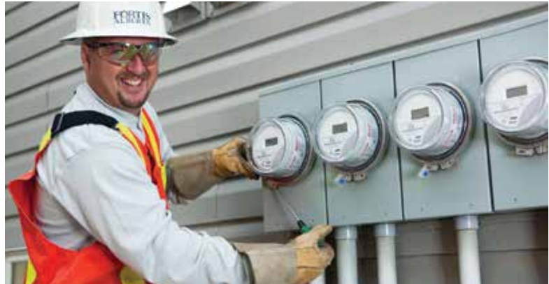
Toronto Power line technician Pete Patton installs an automated meter. Photo courtesy of FortisAlberta Inc.
