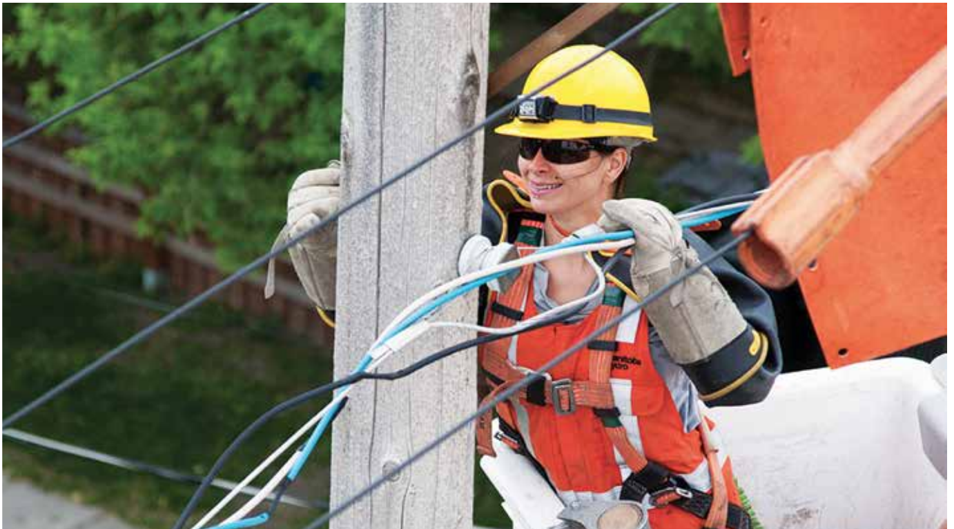
Power line technician, Jessica Hadfield safely repairing a line. Photo courtesy of Manitoba Hydro.
