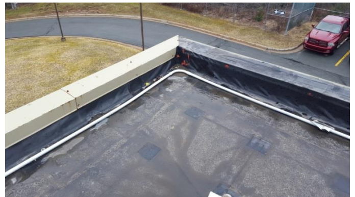
Photo B.16 – Cap flashing removed (north corner).
