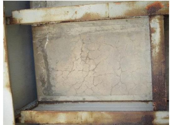
Figure 16: Cracking of concrete deck.
