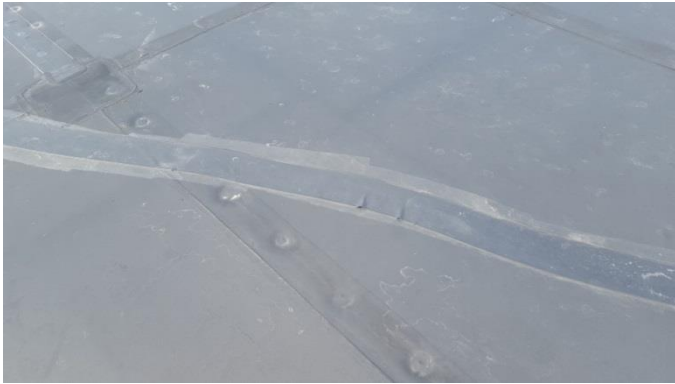
Photo B.55 – Seal edge failure at patch cover strip.
