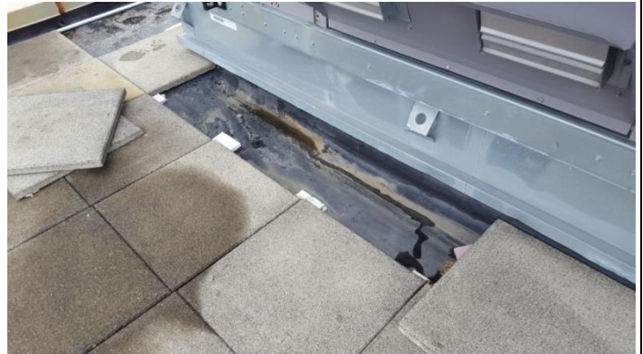
Photo B.26 – Typical buildup at mechanical curb.
