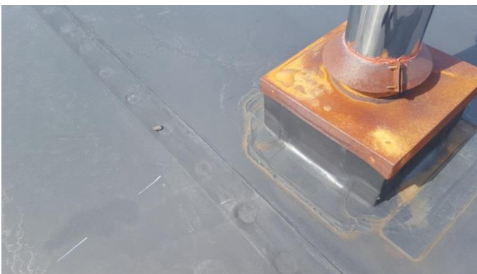
Photo B.29 – Chimney curb with rusting flashing.
