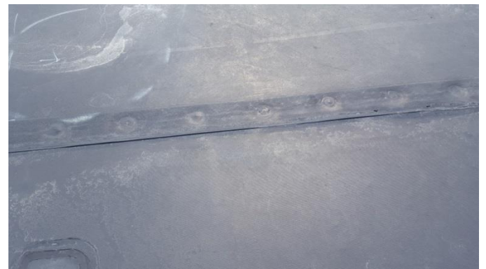
Photo B.28 – Typical original seam with lifting edge.
