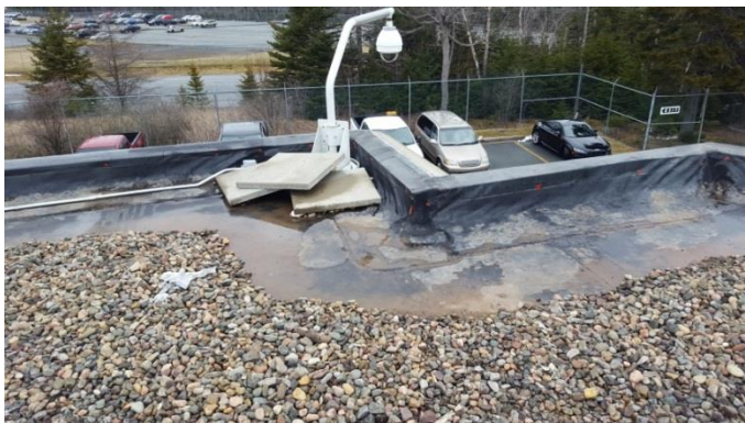
Photo B.9 – Cantilevered light fixture (note ballast).
