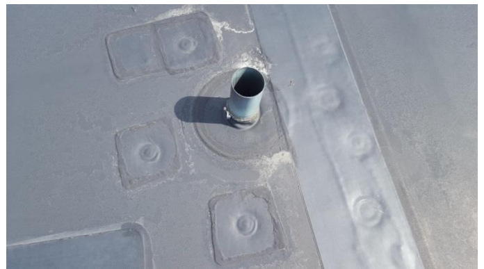
Photo B.40 – Patches over fasteners around vent.
