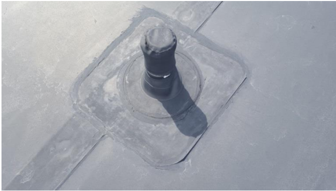
Photo B.61 – Flashing and cover failing at stack.
