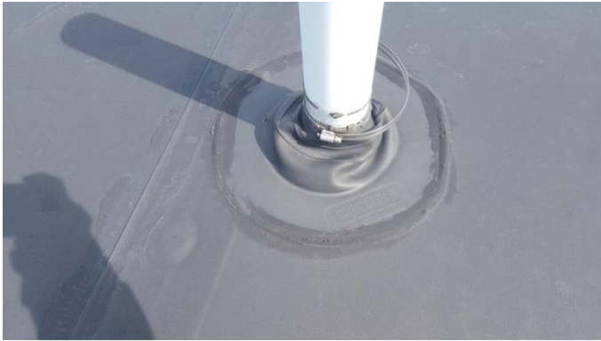
Photo B.37 – Collapsed vent/stack boot (Carlisle).
