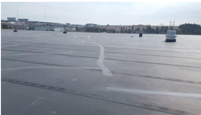
Photo B.57 – Looking showing long patches.
