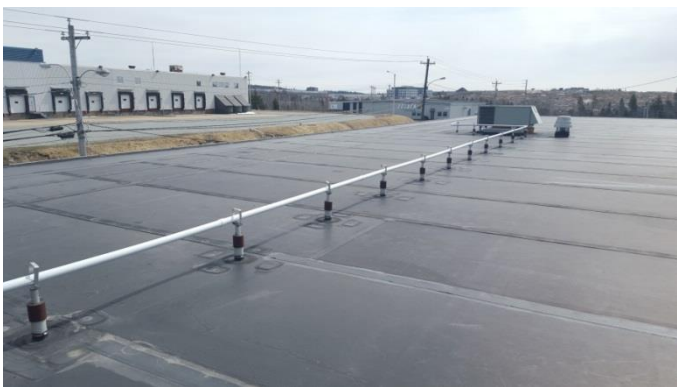
Photo B.53 – Booted mech. pipe support system.
