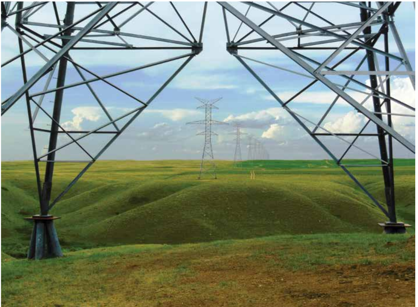
AltaLink's Bowmanton to Whitta Transmission Project—a 240 kV transmission line from east of Medicine Hat to South of Whitta—was built on screw pile foundations. Photo courtesy of AltaLink.
