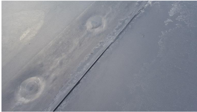
Photo B.31 – Close-up of failing seam.
