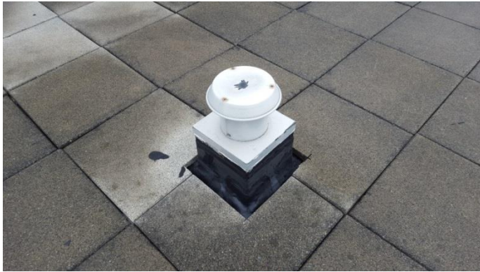
Photo B.25 – Paver trimmed at penetrations, typ.
