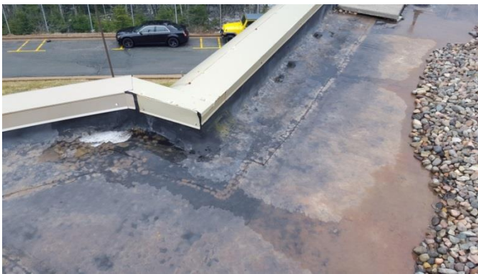
Photo B.33 – Note flashing condition (poor jointing).
