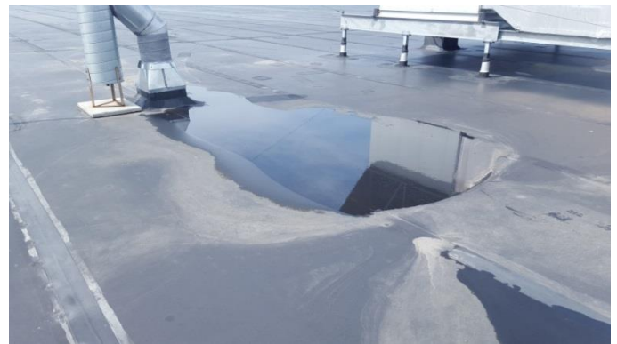
Photo B.52 – Standing water east of AHU (<10mm).
