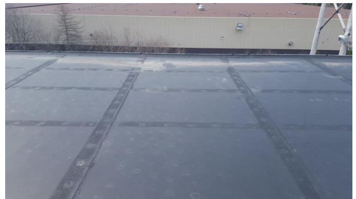
Photo B.58 – Seal deterioration, south end, mid roof.
