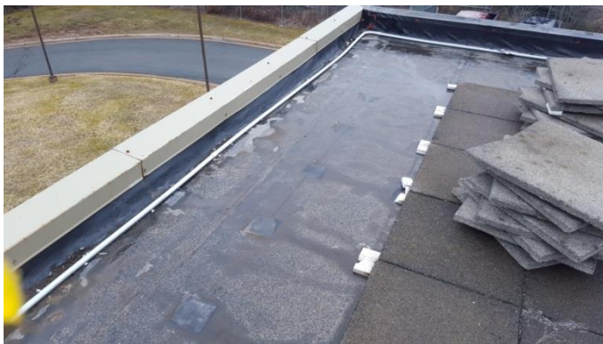
Photo B.17 – Note patch repairs in EPDM.
