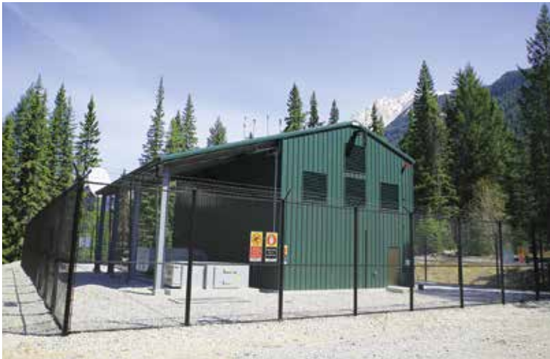
A view of the exterior of BC Hydro and Power Authority’s Field energy storage facility. Photo courtesy of BC Hydro and Power Authority.
