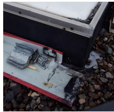
Photo B.40 – Flashing screws and brackets (loose).
