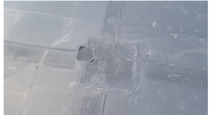
Photo B.32 – Patch lifting due to adhesive failure.
