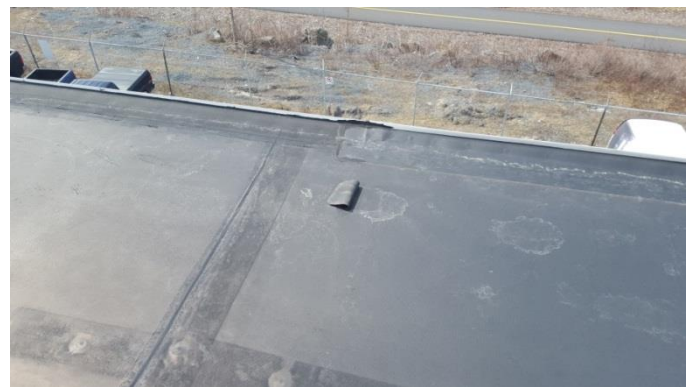
Photo B.60 – Adhesive failure at edge flashing.
