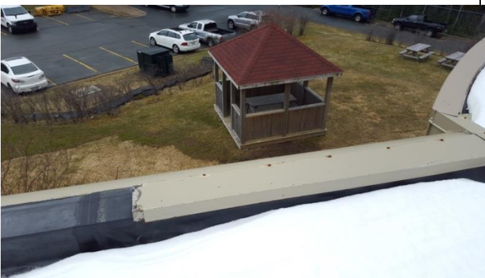
Photo B.35 – Cap flashing not present (south edge).
