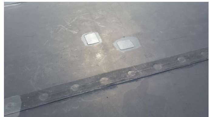
Photo B.34 – Recent membrane patches.
