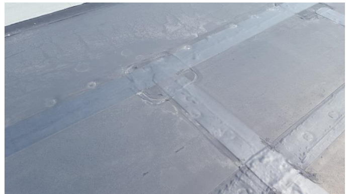
Photo B.16 – Typical seam cover patch intersection.
