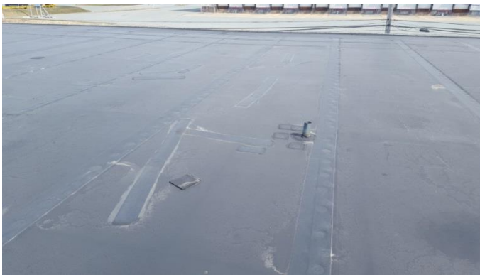
Photo B.39 – Patches at northeast corner of roof.
