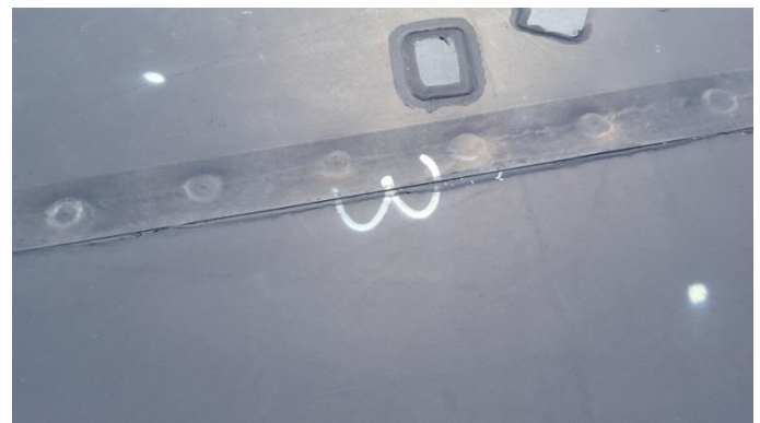
Photo B.36 – Failing adhesive at seams & patches.
