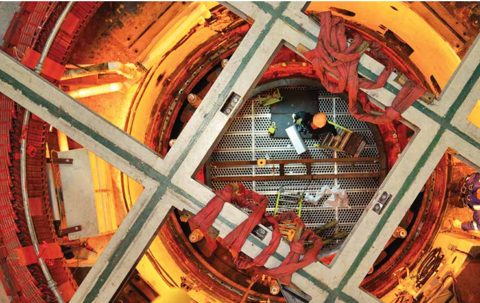
A 10-year maintenance of one of our Whitehorse hydro units. Photo courtesy of Jim Petelski/Yukon Energy Corporation.
