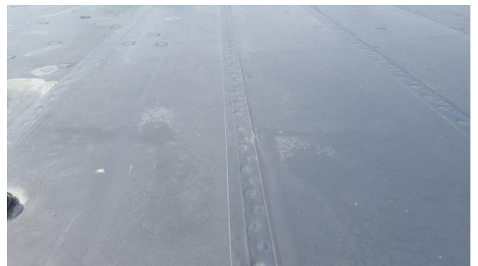
Photo B.22 – Typical seam cover, mid roof near AHU.
