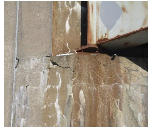
Figure 9: Cracking at northwest bearing seat.
