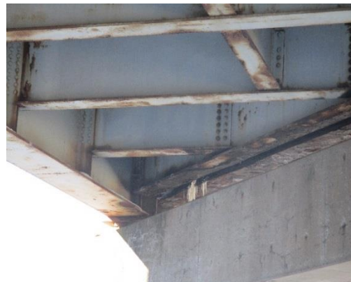
Figure 17: Existing leaky expansion joints. Icicles observed on day of inspection.
