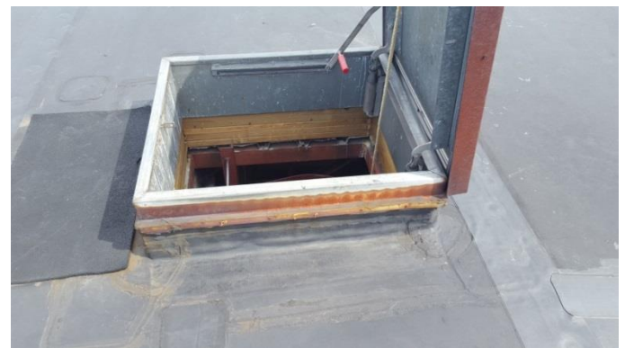
Photo B.66 – Insulation thickness blocking at hatch.
